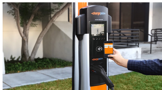
Image depicts a level 2 AC ChargePoint charging station for EVs. (Photo: ChargePoint)
