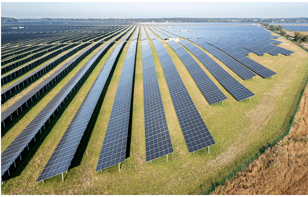
Image depicts EnBW Solarpark Weesow-Willmersdorf, Germany's largest solar park without state funding with 187 MW. (Photo: Paul Langrock, EnBW)
